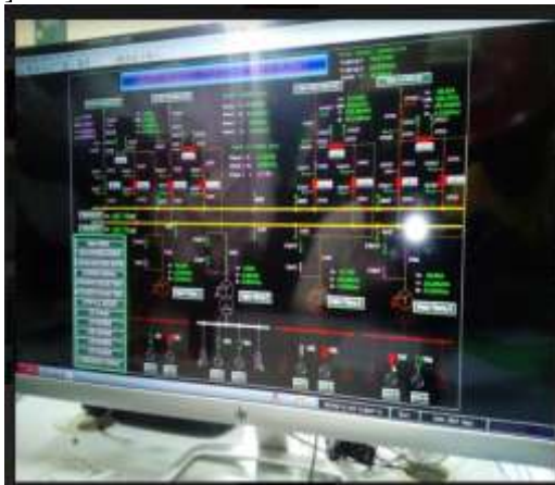
Fig. 3.0: A Snapshot of bus-bar and lines connectivity on Supervisory Control And Data Acquisition (SCADA) system in Olorunsogo phase I Gas Turbine Power Plant.
