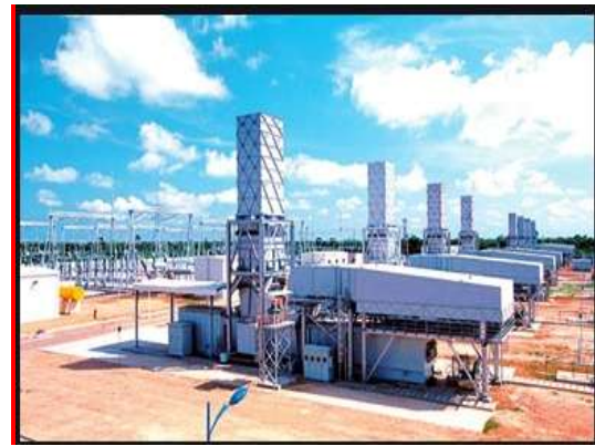
Fig.1.0: Pictorial view of Olorunsogo gas turbine power plant
