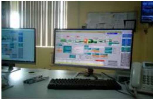
Fig. 2.0: A Snapshot of the Supervisory Control And Data Acquisition (SCADA) system being used in Olorunsogo Gas Turbine Power Plant.
